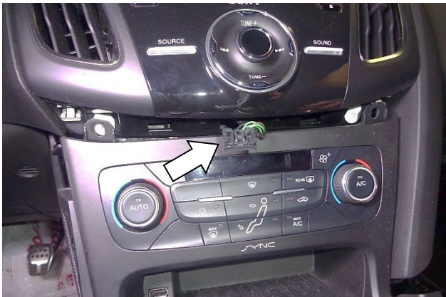
58. Ensure that the center panel bezel plug is exposed and accessible before reinstalling the power panel.
